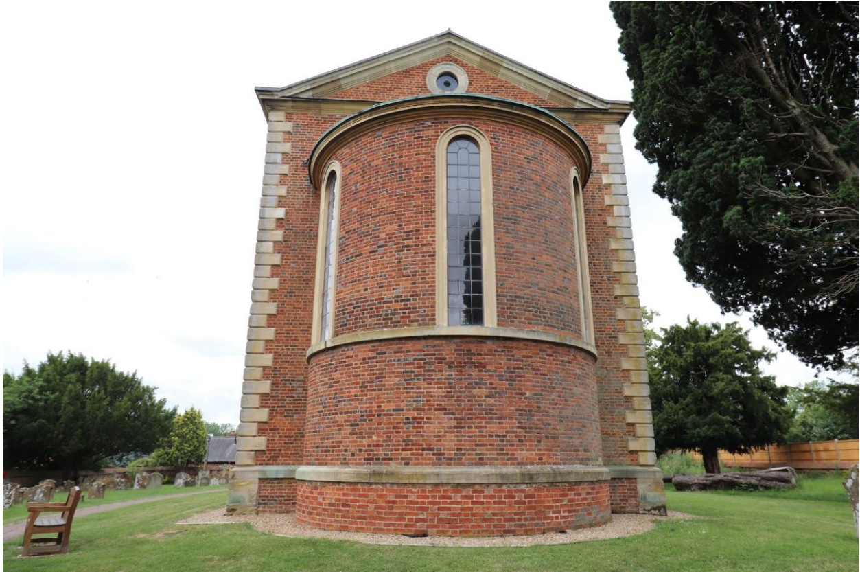
Above: East elevation of the church with apse of c. 1862. Note the different brick below plinth level
