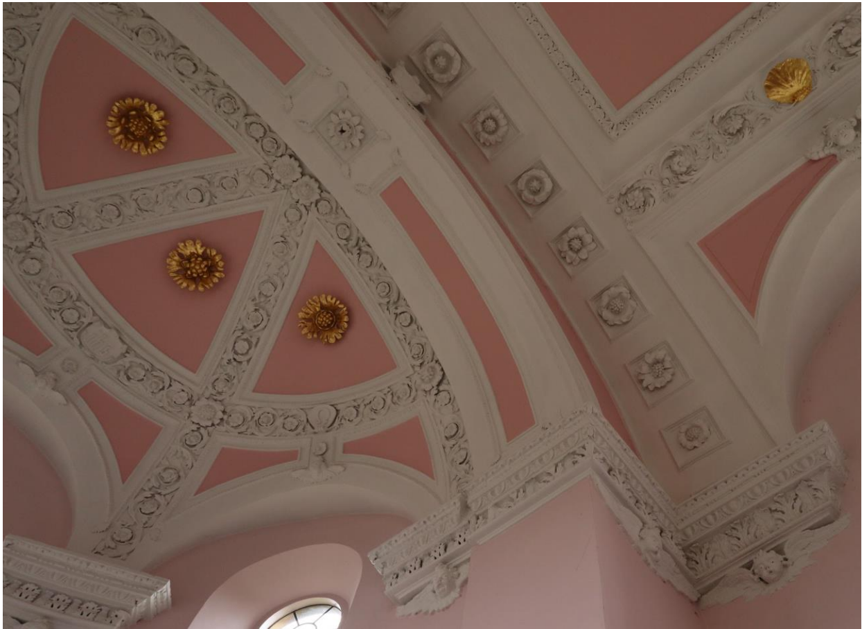
Above: Junction between the nave and apse showing the subtle differences between the plasterwork decoration
