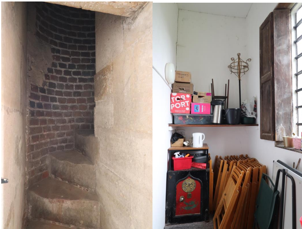
Above left: Stairs to the bell chamber rising through the thickness of the wall
